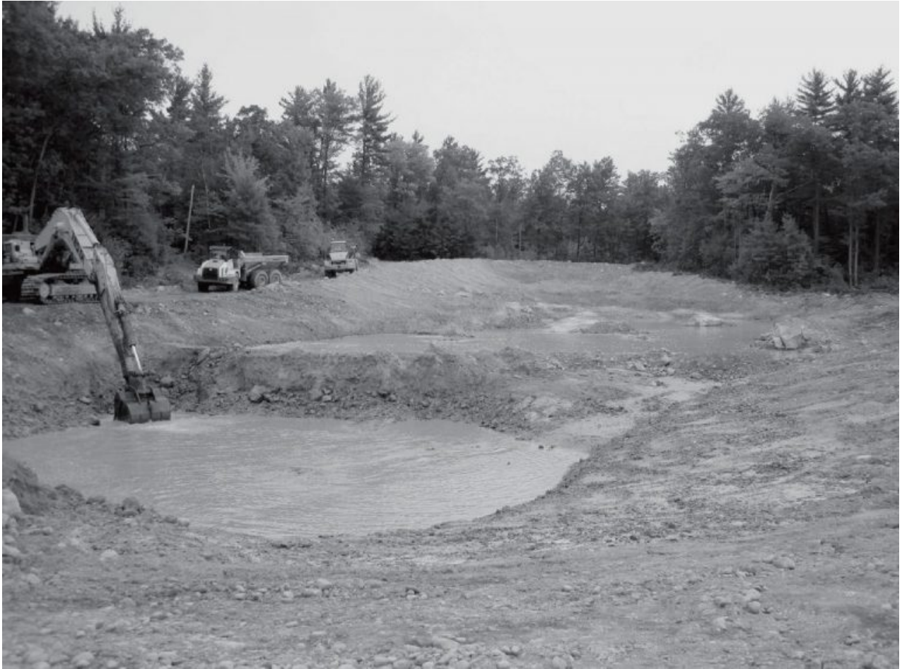
An excavator digs in to make room for more water at the Norco pond. Submitted photo
