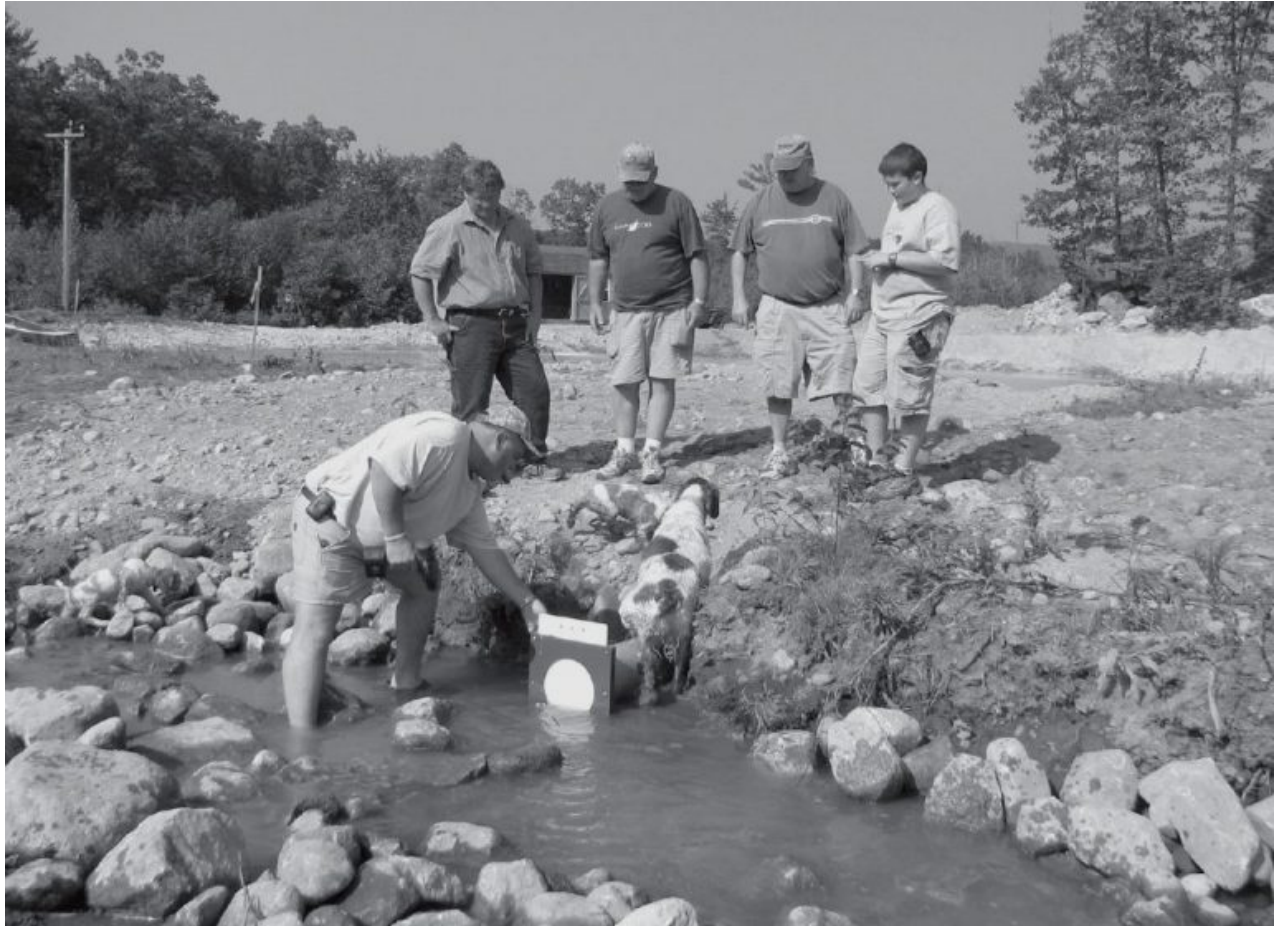
Front, Kevin McManus installs a lock on the gate valve that will be used to raise and lower the level of the water in the event of a major rainstorm at the new pond. Rear, Mike LaFountain, Dick Fontaine, Jack Lynch and Ryan McManus supervise. Phyllis Booth photo
